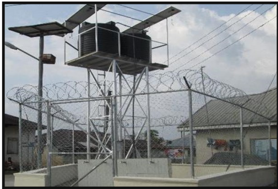
Solar powered borehole water at Mbarakom, Akamkpa LGA
